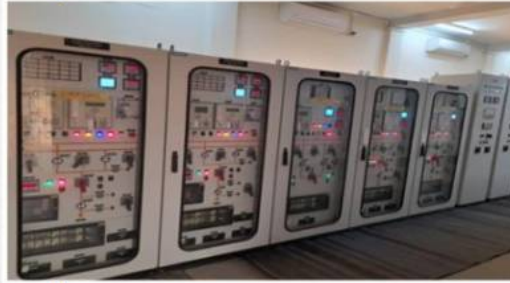
220/33 kV Substation at Amguri, Assam, India
