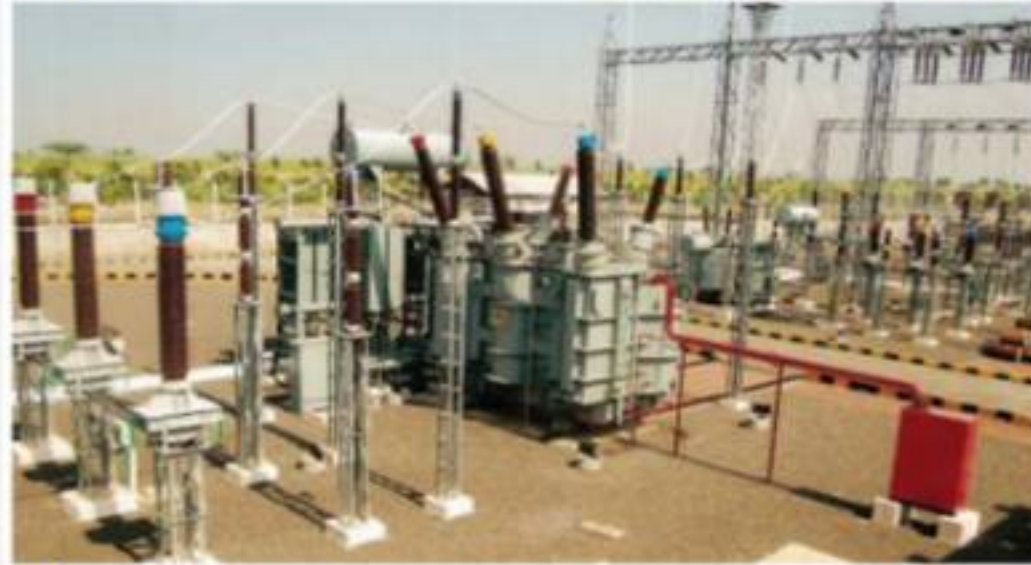
110/11 kV Substation at Koppal, Karnataka, India
