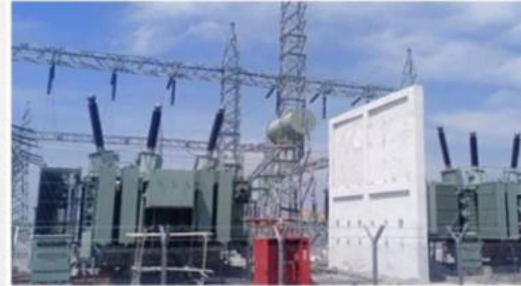
230/33 kV Substation at Thoothukudi District, Tamil Nadu, India
