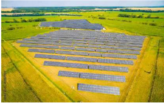
Utility Scale Solar-Storage Turnkey and BOP EPC solutions
