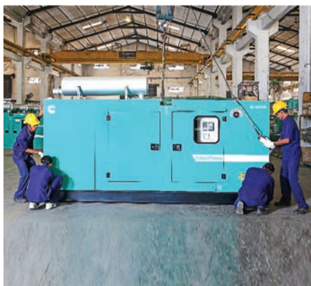
DG Set Manufacturing Unit Phaltan, Maharashtra
