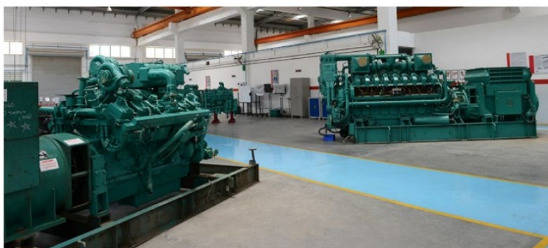
Demand will stay in high voltage capacity genset
