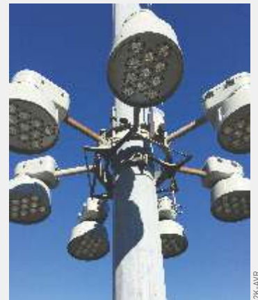
High Mast Lighting
