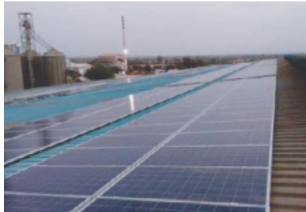
540 KW at Adani Group, Rajasthan
