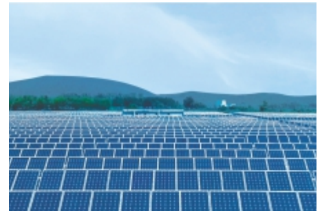
65 MW NTPC Limited, Rajasthan
